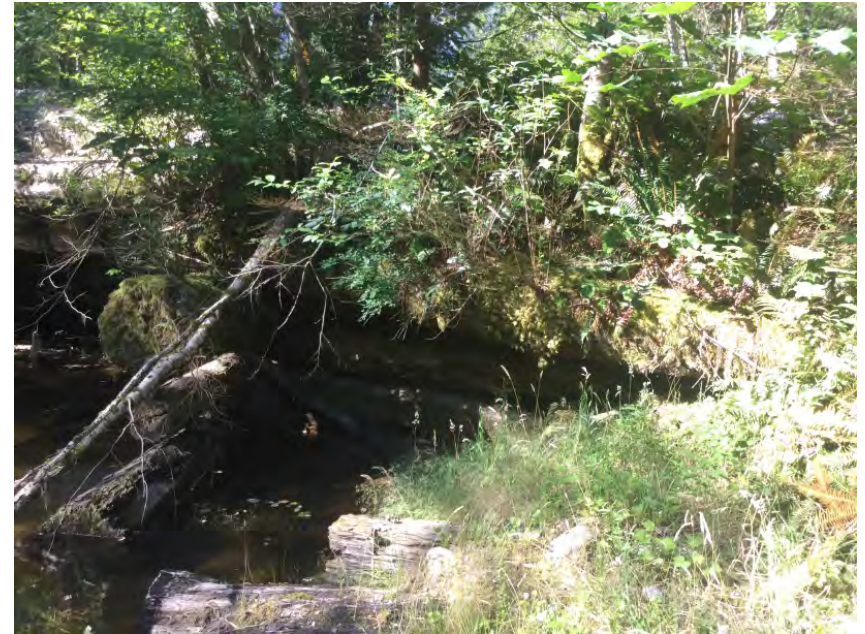
Possible Scour at Left Abutment Upstream Corner.
